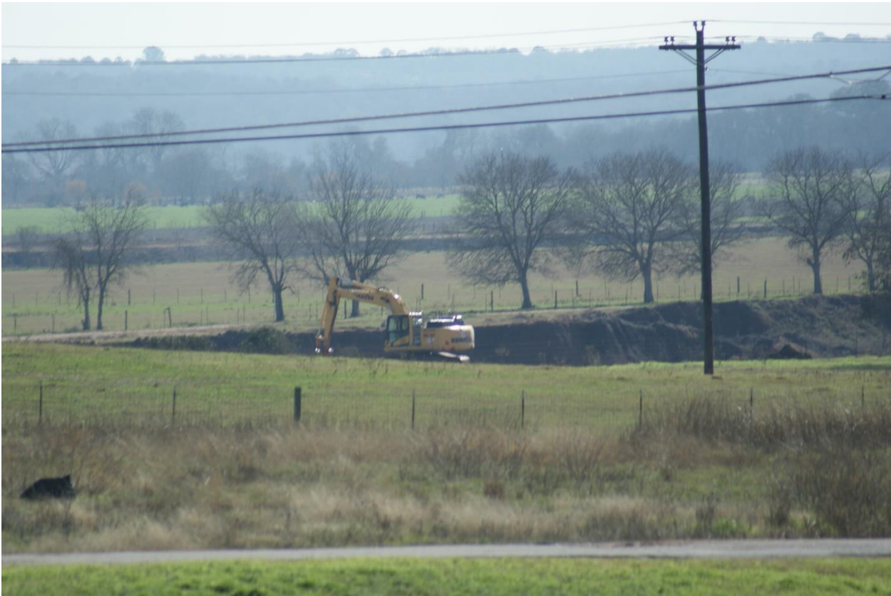
Figure 5. Newest sand pit from the Stop Sign outside Mike D's house\
